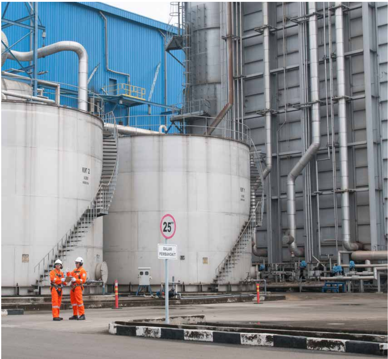
▲ Oil Tanks di PLTGU Jababeka Oil Tanks at GSPP Jababeka
