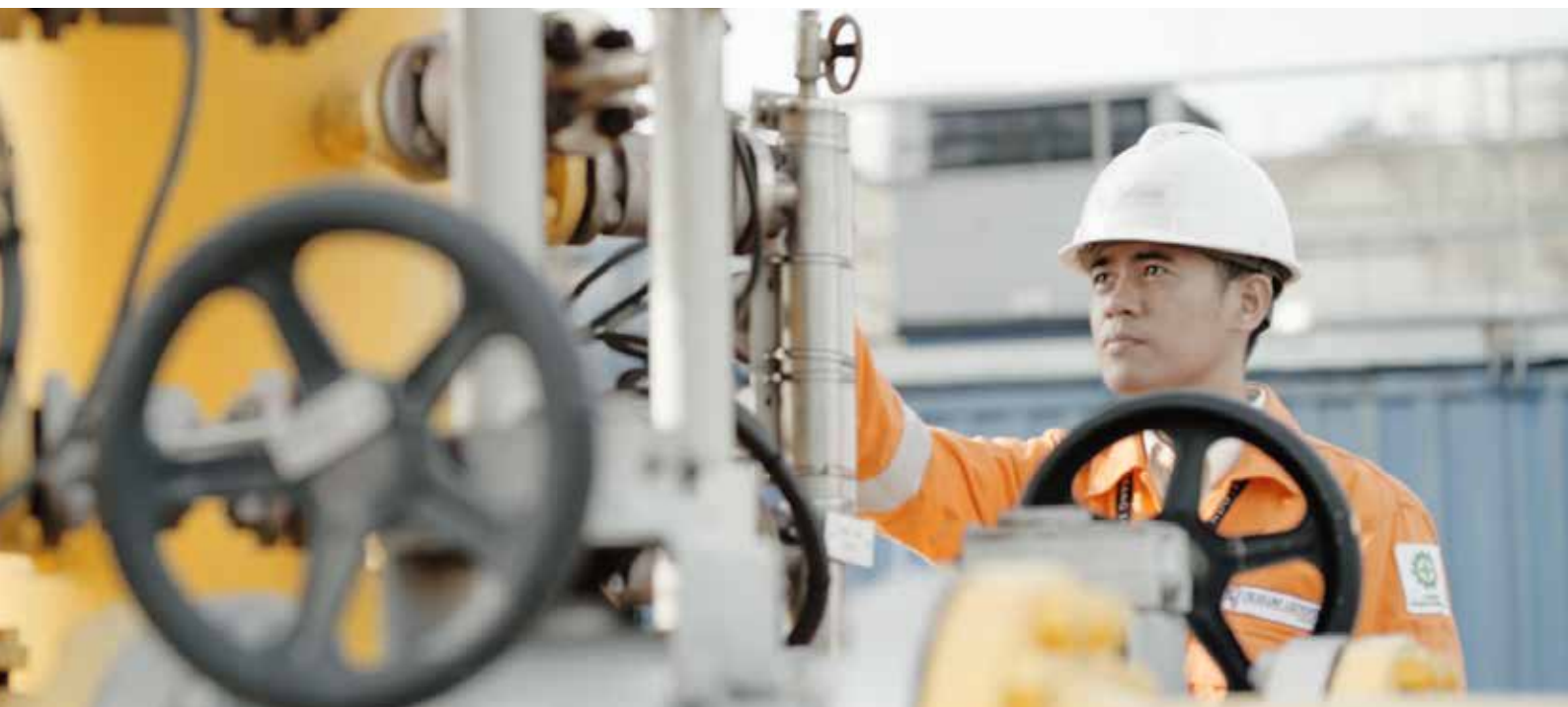
▲ Flue Gas Coalescing Filters di PLTGU Jababeka Flue Gas Coalescing Filters at GSPP Jababeka
