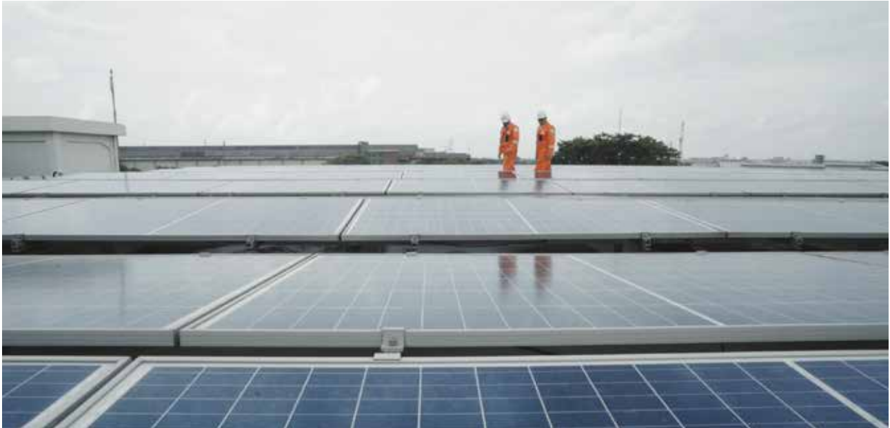
▲ Panel Solar Rooftop Solar Rooftop Panels
