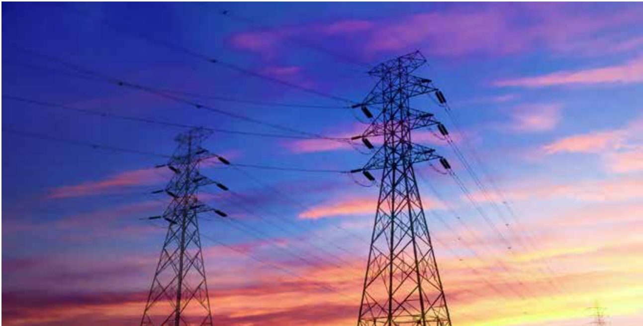
▲ Menara Transmisi 150kV 150kV Transmission Towers
