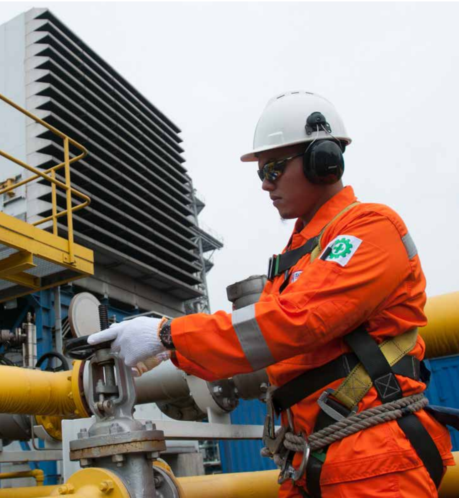
▲ Gas pipeline di PLTGU Jababeka Gas pipeline at GSPJ Jababeka
