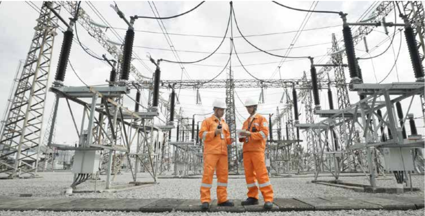
▲ Switchyard di PLTGU Jababeka Switchyard at GSPP Jababeka
