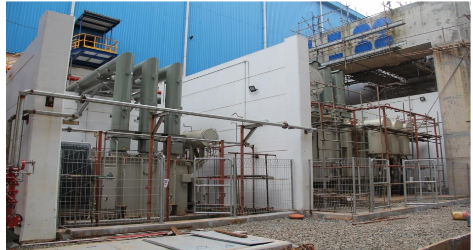
1BAT10 and 1BBT10 Transformers
