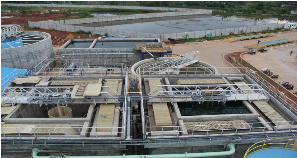
WTP Clarifiers, Sludge Thickener, Centrifuge, Belt Press and PH Correction Tank
