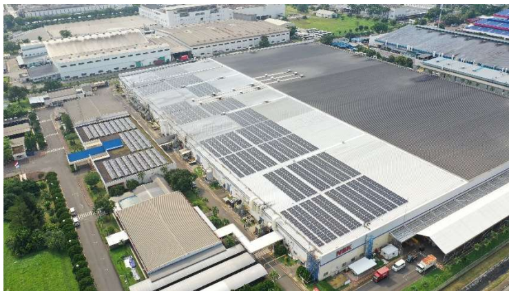
PLTS Atap di atap pabrik PT NSK Bearings Manufacturing Indonesia sebesar 1 MWp
