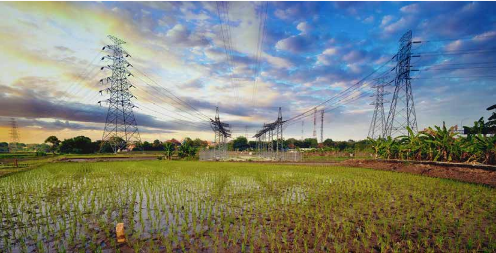
🕒 Jalur transmisi bertegangan 150kV 150kV transmission lines
